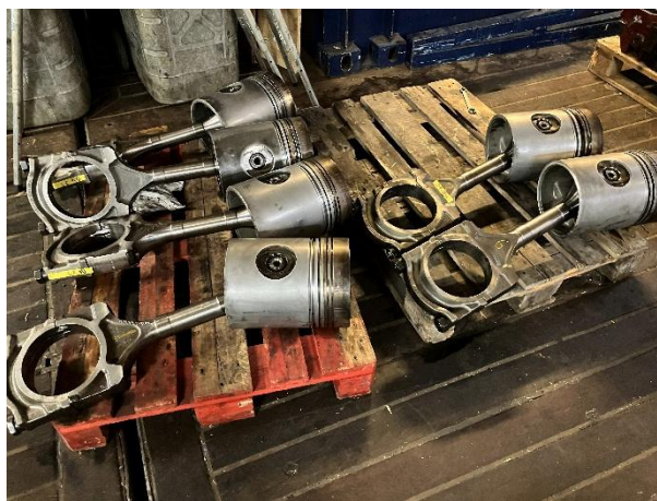
Figure 2: Removed pistons of the diesel generator under repair, of which a total of 4 machines form the heart of the ship (© G. Bohrmann).
